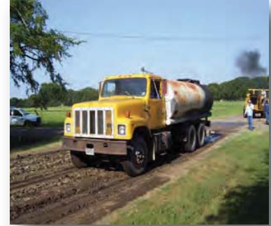
3) Pre-water disturbed road.
