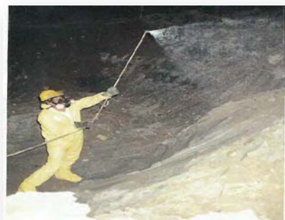
Hazardous Site Sealing
